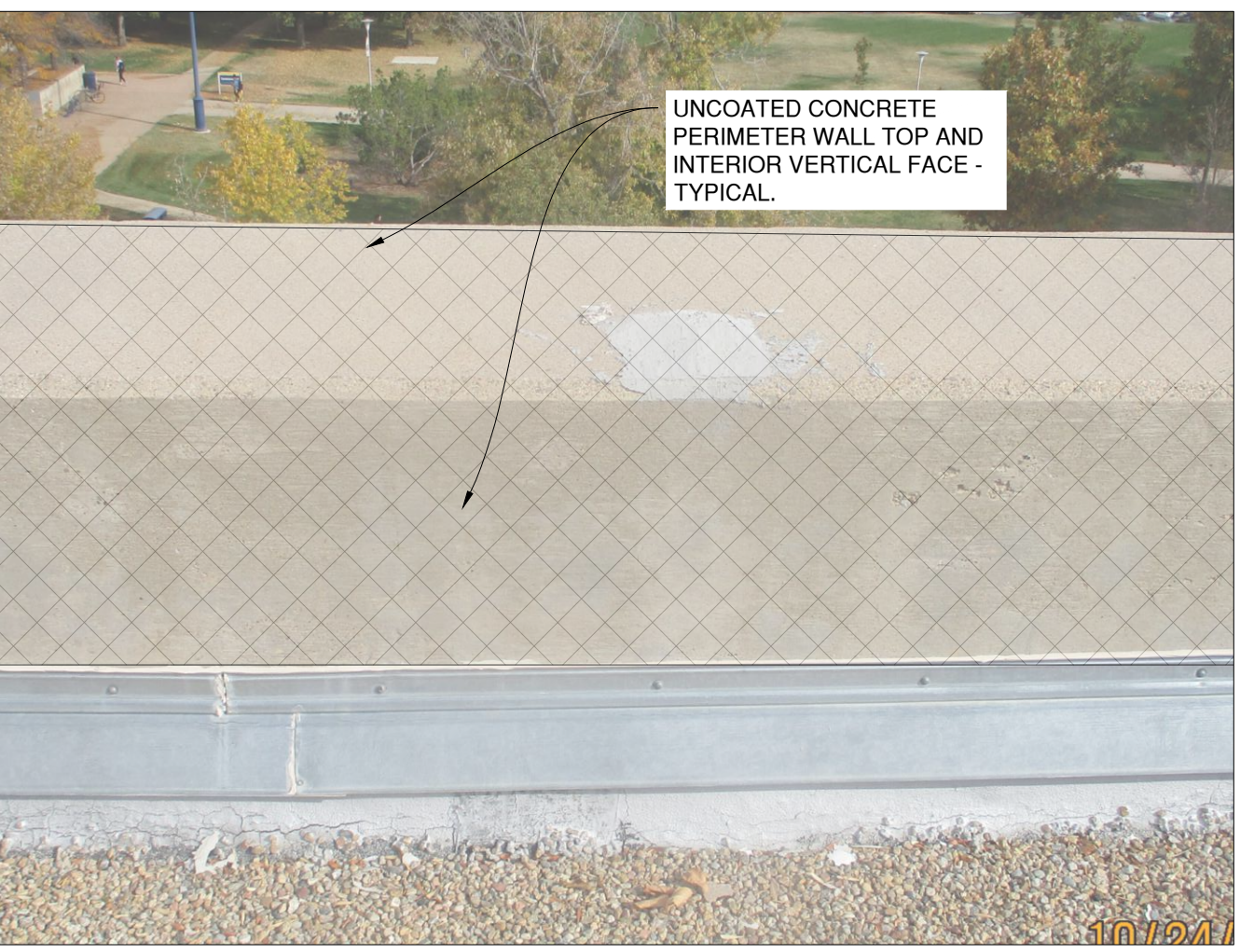
F UNCOATED PARAPET WALL - TYPICAL NOTE: SIMILAR - ACTUAL CONDITIONS MAY VARY (N.T.S.)
